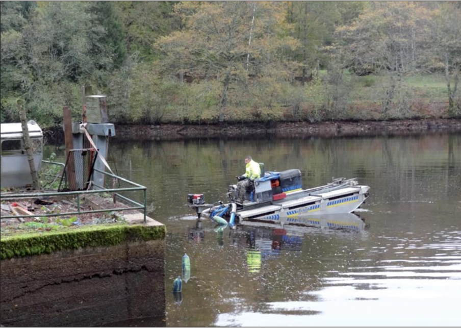
[5] Pumping bottom deposits from the Chailloux pond with an amphibious barge equipped with a suction pump
